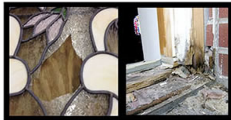
broken glass deteriorating frames
